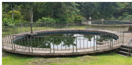
Vailima Water Treatment Plant
