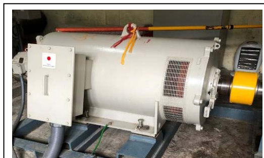
Bajhang Micro-Hydropower Station's Generator
