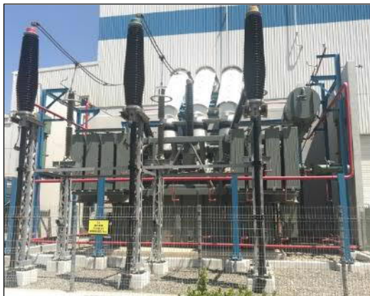
Left photo: Main transformer
