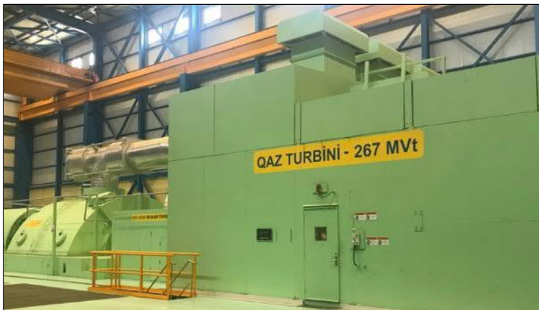
Left photo: Steam turbine (back left) and gas turbine (front)
