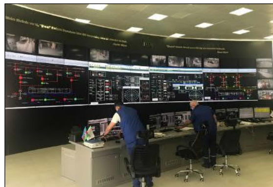
Right photo: Control room
