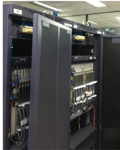
Interface equipment installed in the Project
