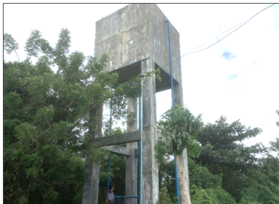
Photo 3: Established Water Supply Facility (Ilocos Norte Province)
