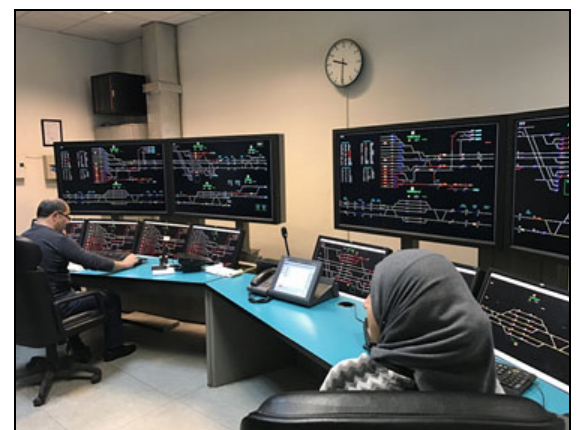
Operation Control Room with equipment procured by the Project
