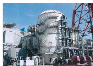
Flue Gas Desulfurization
