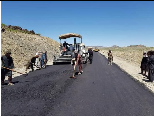
Asphalt improving works as part of Periodic maintenance at the Road site
