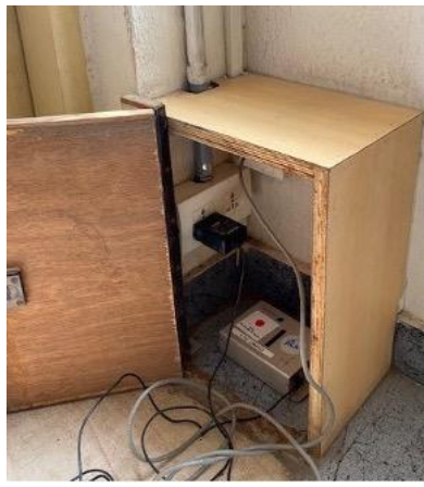
Strong motion sensor (ITK sensor) installed in the IIITH building to conduct constant monitoring
