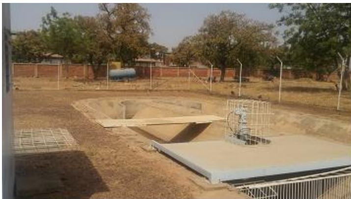
The pilot high-speed algal channel wastewater treatment plant in the campus of Kamboinsé, 2iE
