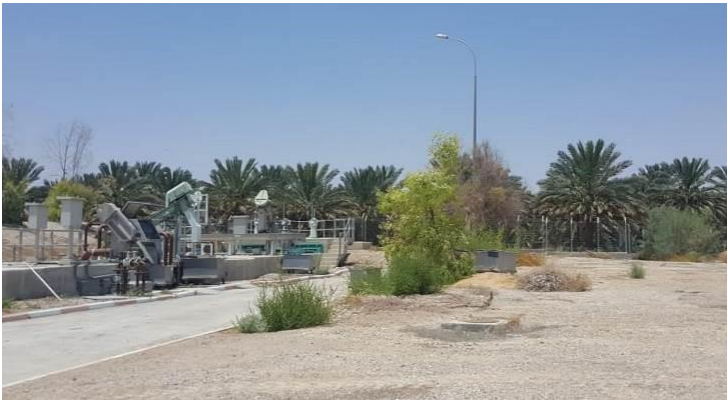
Treated water is kept in the pool and is supplied to dates farmers, who installed pumps along the pool.
