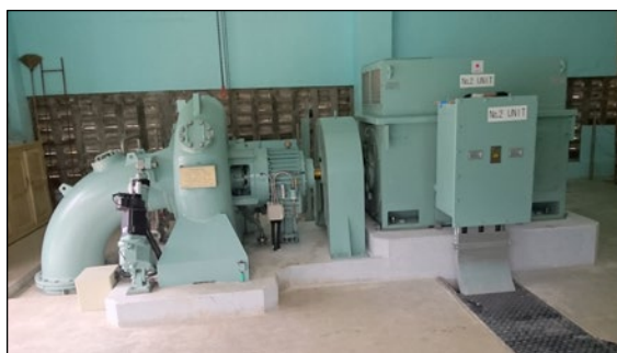
Water Turbine and Generator
