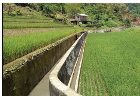
Headrace. The narrow canal on the valley side is the rehabilitated irrigation channel.
