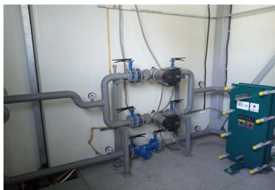
Photo 4: Connection pipes of pellet boiler (Kindergarten in Cricova)
