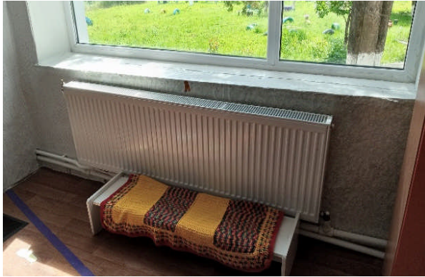
Photo 1: Heating system utilizing pellet boiler (Kindergarten/cultural facility in Furceni)
