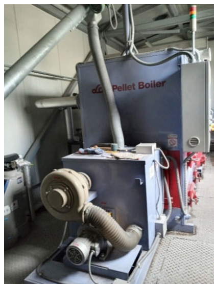
Pellet boiler introduced by this project
