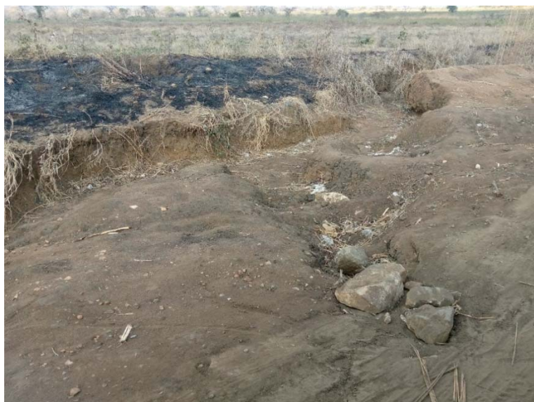
Photo 1. Example of road condition between Magige and Cuamba
