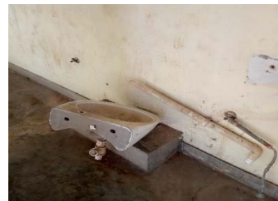
Damaged toilet sinks
