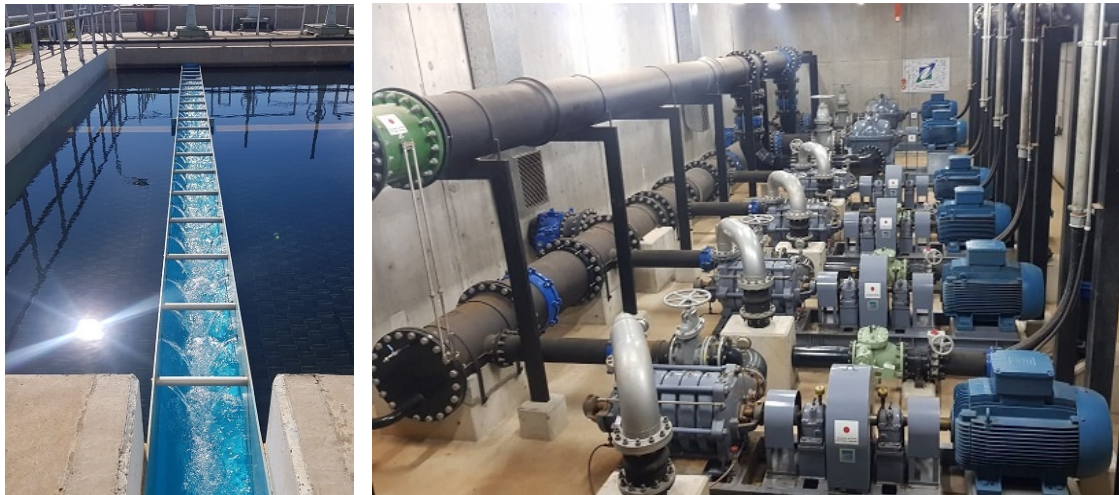
Water Treatment Facility (left) and Pumping Facility (right) of the New WTP
