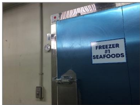
The replaced door of a freezer (Castries)
