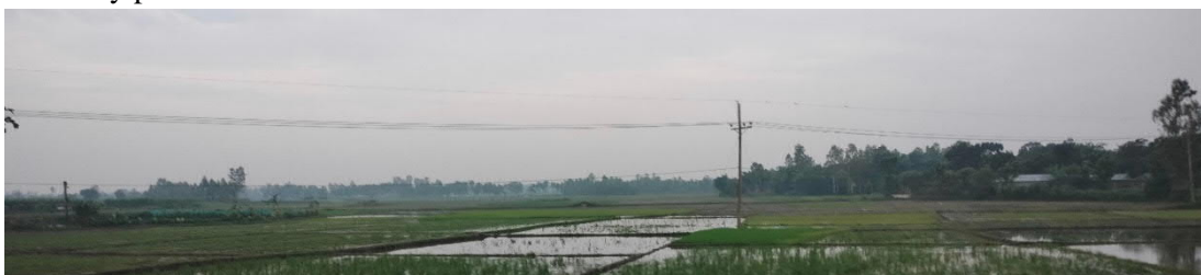
Photo Newly Constructed Medium- and Low-Voltage Lines (33 kV Line) (Rangpur Division, Dinajpur PBS-2)
