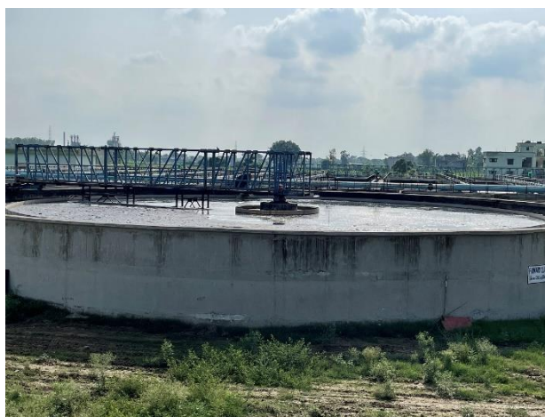
Sewerage treatment plant (Settling basin)
