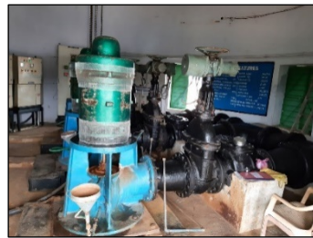
Pumping Facility (Tiruchirappalli)
