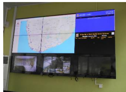
Equipment procured for the information-display system
