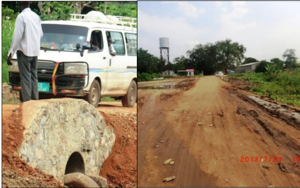
A new culvert (left) and a road after repair can be driven straight through. (right) (September 2013) source: Project Team
