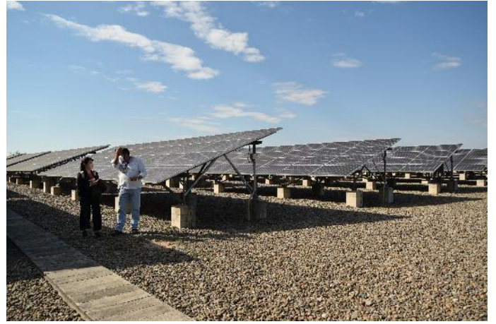
Solar panel installed at AASANA.
