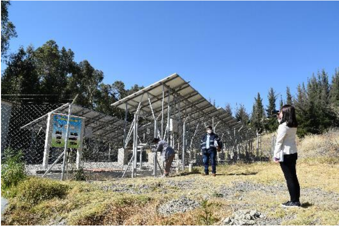
Solar panel installed at UMSA.
