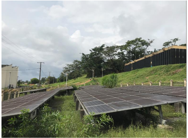
Solar panels installed at UOB
