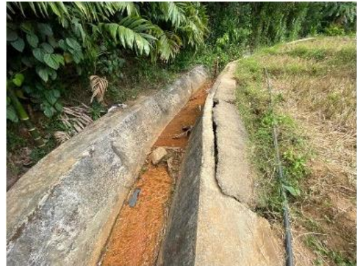
(Drainage, Udamadura, Nuwara Eliya) Damaged and need to be repaired.
