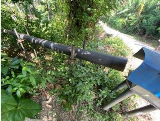
(Extensometer, Udamadura, Nuwara Eliya) Damaged and need to be repaired.
