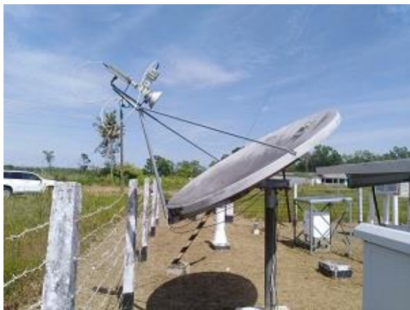
V-SAT of Aralaganvila Station
