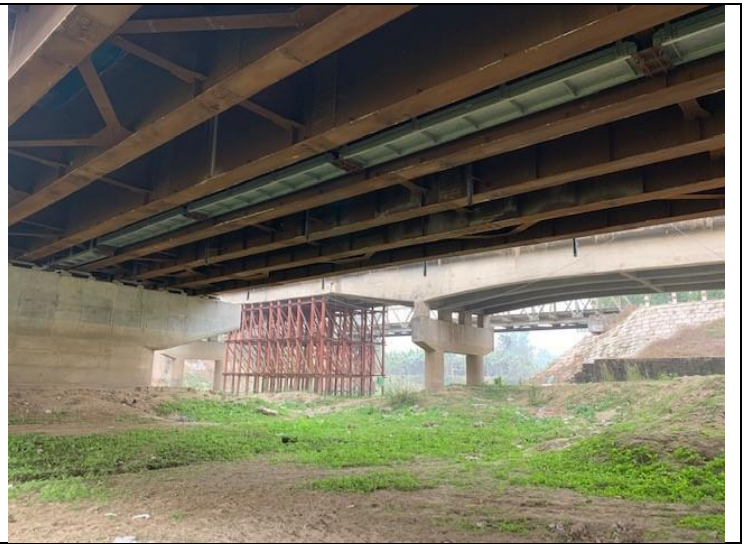
Site visits at Mohosthan Bridge (old bridge with retrofitting and new bridge)
