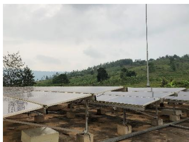
Solar panels for pump operation
