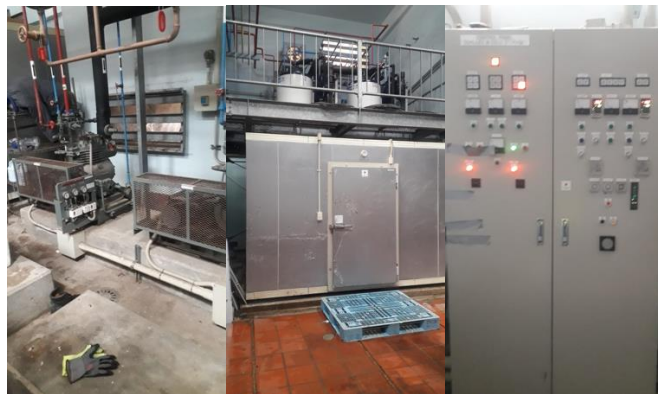
Compressor system, ice maker with drums, and control panels at Grenville Fisheries Complex
