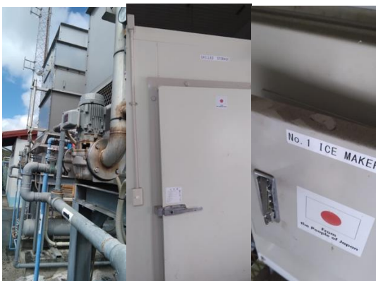
Tower and pump of the evaporative condenser, chill room, and ice maker at Melville Street Fisheries Complex
