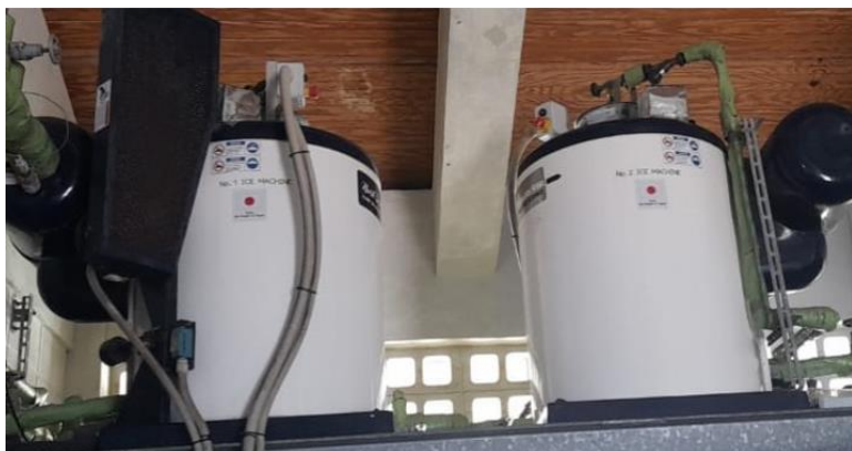
Ice-making machines installed at Union Island Fisheries Centre (Clifton) under this project. Photograph taken on the January 14, 2022
