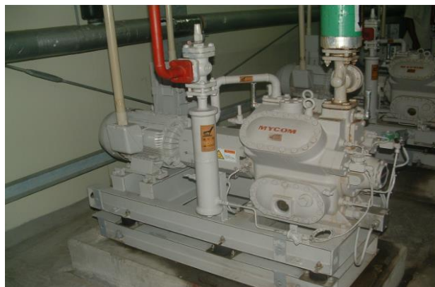
Ice-making machine compressor overhauled in 2016 under this project at Kingstown Fisheries Centre. Photograph taken on August 16, 2021
