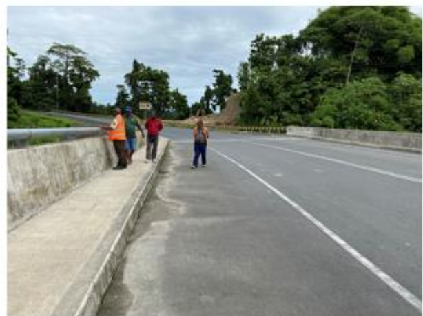
Curbside walkway has been installed on the Aum Bridge (Source: External Evaluator)
