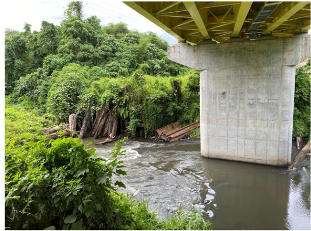
Unimplemented revetment works of the Aum Bridge (Source: External Evaluator)
