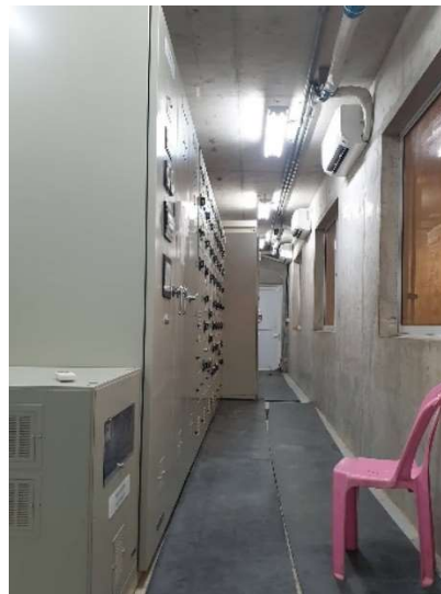
Distribution Pump Station Control Room
