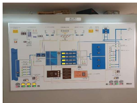
Water Distribution Flow Monitoring Panel
