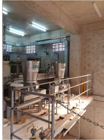
Chemical Feeding Facility
