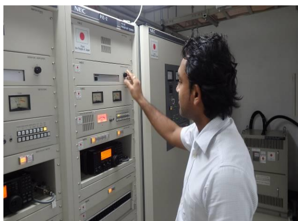
MW Radio Broadcasting Equipment procured under the project
