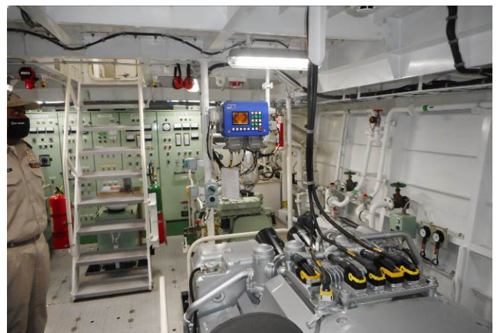
Starboard engine (bottom right) and its control panel (back)
