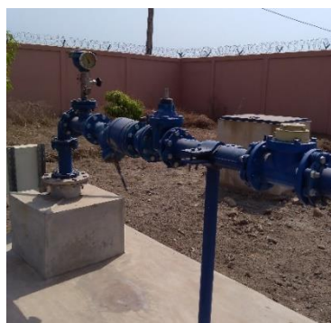
Water Source Facility at Dassa-Zoume (3-SE8) (Photo taken by the evaluator)
