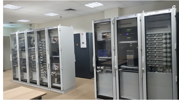
Multiplexer (MUX), inverter, etc. inside the MERCC
