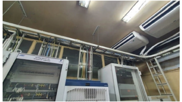
Photo 2: Communication Equipment, Air Conditioning Equipment (UERCC)
