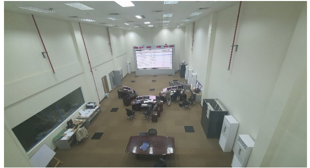
Photo 4: Control Room (MERCC)
