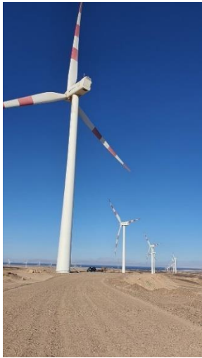
Photo 3: Wind Power Generator
