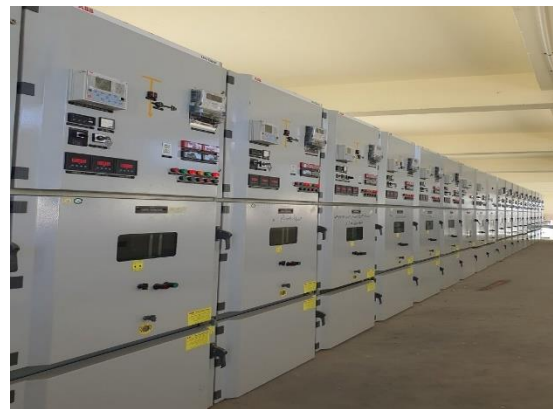
Photo 2: Switchgear for Power Distribution (EETC Facility)
