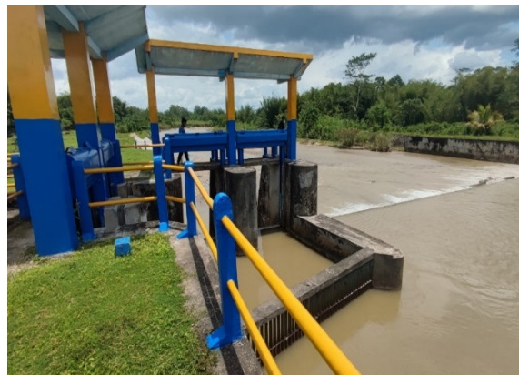
Developed Intake Weir (Way Apu Subproject)
