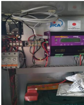
Automatic Water Level Recorder installed in BWS Sulawesi I.
