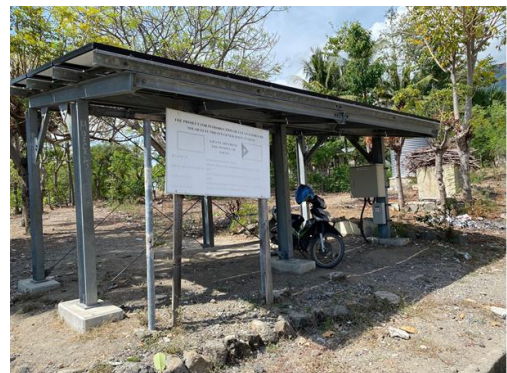
Stand-alone PV system at Atauro Basic School (The roof part of this facility is a PV panel)
