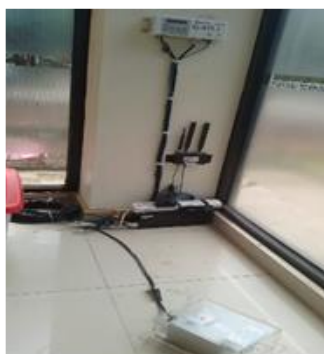
Installed IT seismic intensity meter (Source: photo taken by the evaluator)
