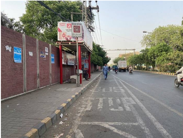
Signboard for bus stop relocated and word marking "BUS STOP" installed by TEPA according to Action 1 of the TMP
