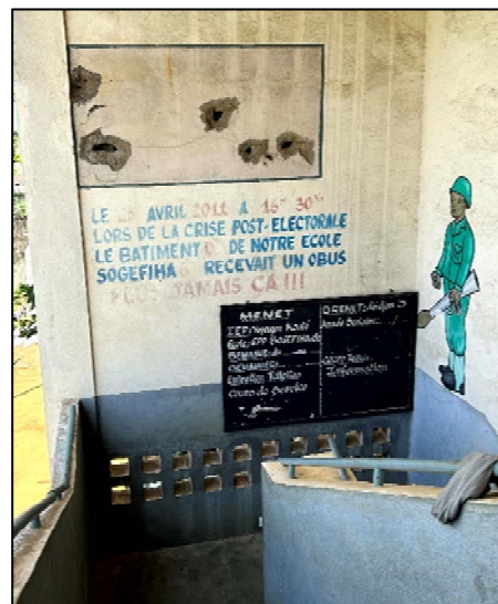
Photo 1 School Renovation Pilot Project in the Commune of Yopougon. The Mural Showing the Scars of the Conflict. Source: Photo taken by the evaluator.
