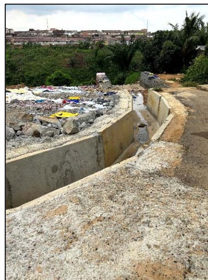
Photo 6 Reinforced Endpoint of Drainages by Phase2 (Abobo) Source: Photo taken by evaluator.
