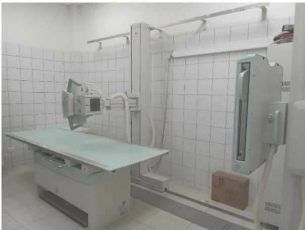
X-ray device installed in the Lepaera Health Facility.
