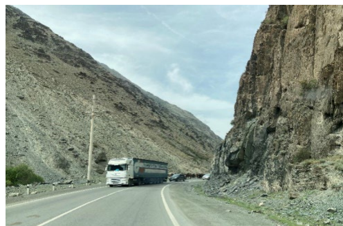
Landslide and rockfall hazard area on the Bishkek-Osh Road (source: Evaluator)
