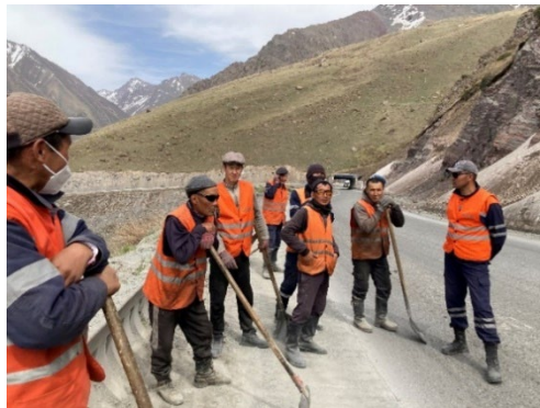
DEP staff engaged in maintenance work near the snow fence (Source: Evaluator)
