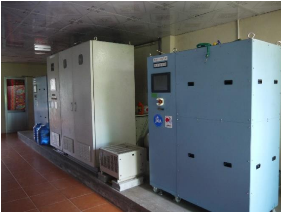
SOFC system and distribution control panel installed at Demo-site, Ben Tre province
