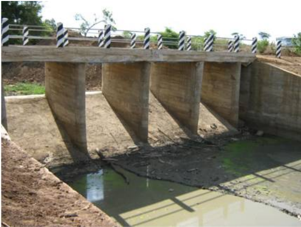
Intake Wier at Kasese Irrigation Scheme (Mwankulu Village)
