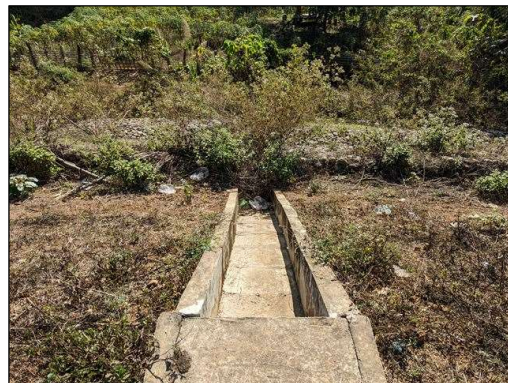
Drainage Ditch in the Approach Road (Filled with weeds and trash)
