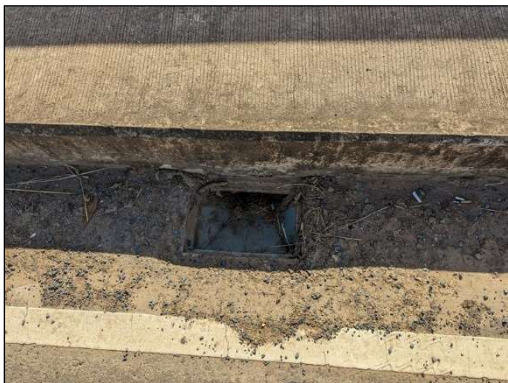
Drainage Hole in the Main Bridge (Lid is missing)
