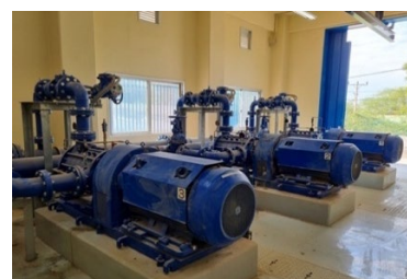
Ma'adi Pump Station
