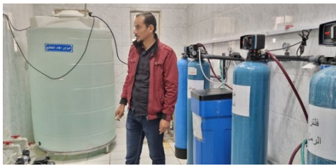
Water purification plant for dialysis rooms, sterilization rooms and laboratories
