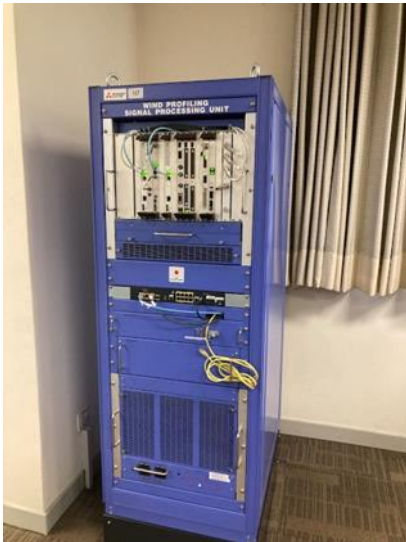
Picture 1: Wind Profiler System (partial) (Inside the PMD Islamabad Meteorological Radar Tower) (Source: picture taken by the evaluator)
